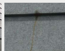
Example of rust
