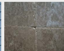
Example of chipping
